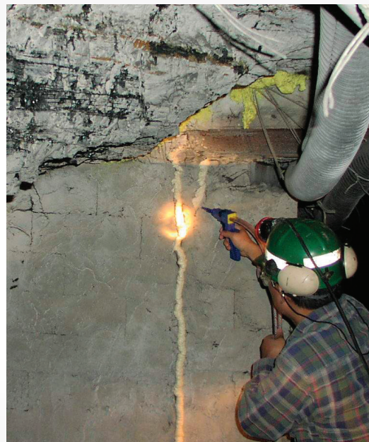
REPAIR DAMAGED BLOCK STOPPINGS
